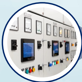
POWER DISTRIBUTION SYSTEM
