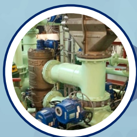
BALLAST WATER TREATMENT SYSTEM
