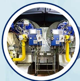
BOILER AUTOMATION SYSTEM
